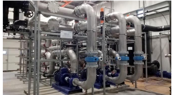
WWTP BIOCOM Nesvizh, Ultrafiltration
